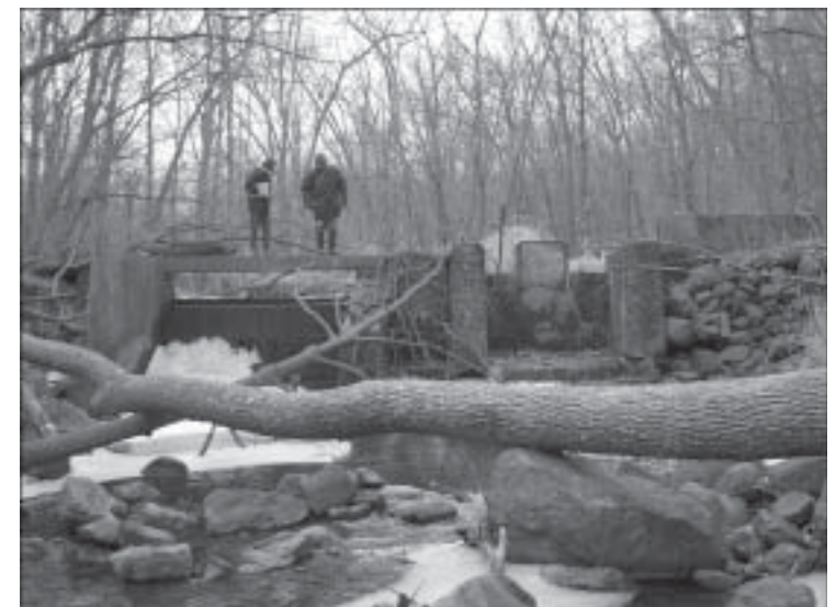
One of the Boulder Creek dams that was removed this past July. Photo courtesy of Cailin Orr
